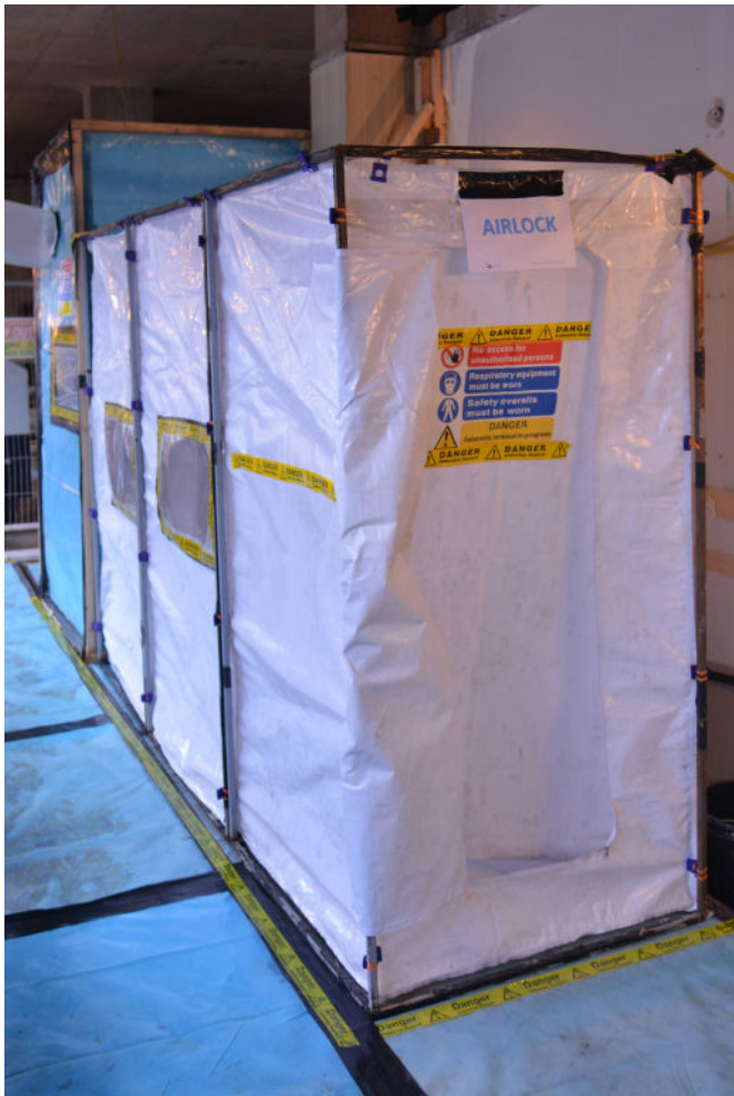
Figure 4: Licensed asbestos removal work has its own specific standards for creating AMBER exclusion zones – signage on a 3-stage airlock
