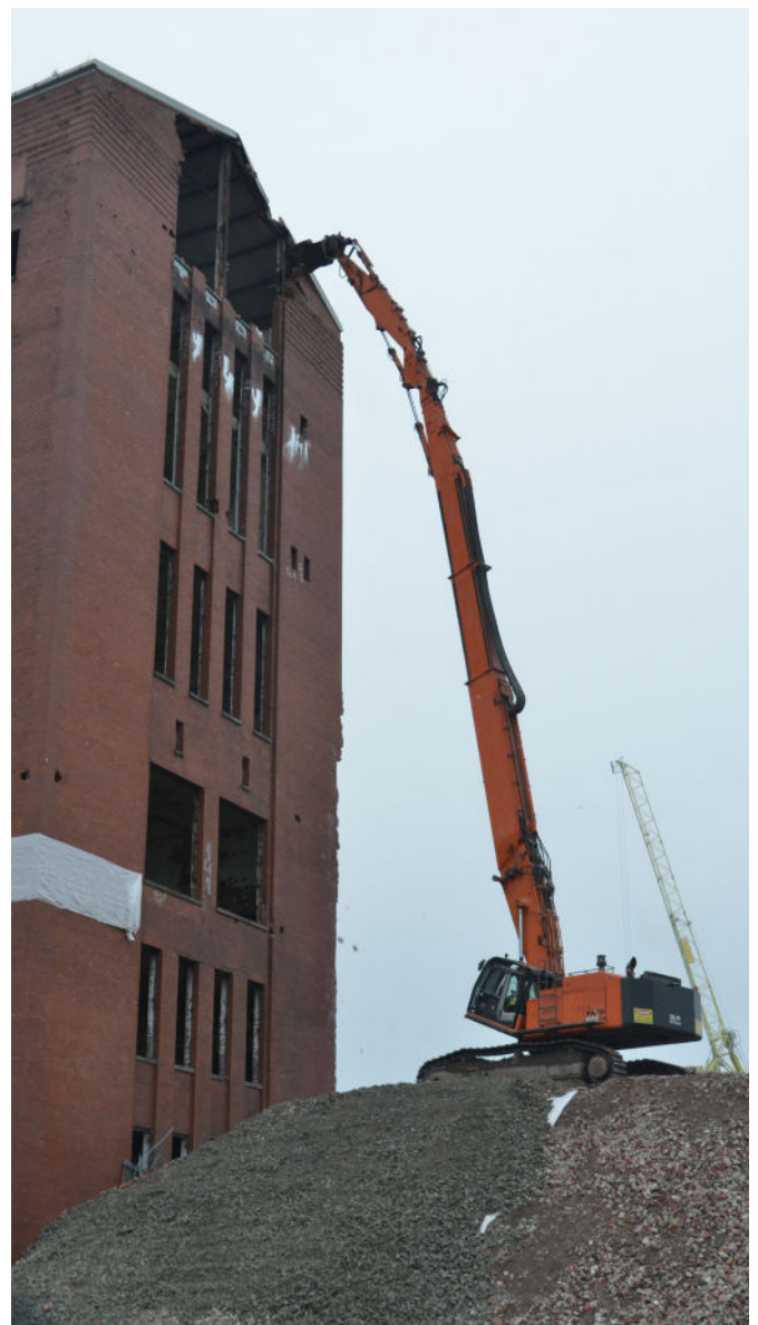
Figure 9: A high reach demolition machine using a ramp as protection from debris and to gain reach
